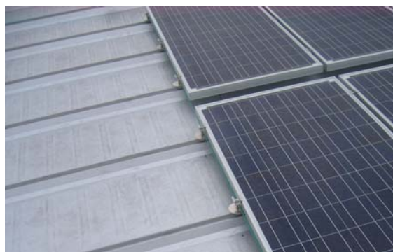
The solar panels were attached to the MR-24 roof panel seams, eliminating the need for roof penetrations and ensuring the continuation of the roof's 25-year weathertightness warranty.
