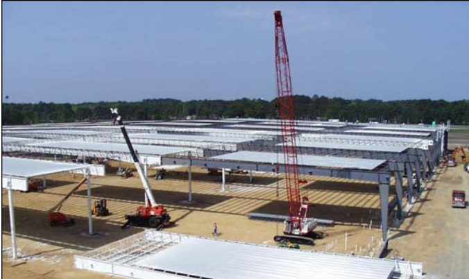
The JCB manufacturing facility for heavy industrial equipment features forty 50'x140' bays erected by BES. Twenty of the bays were ground assembled—including the decking and 3-3/4" Thermax—and then lifted onto the columns.
